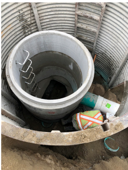
New 1350mm overbuild manhole installed at 225 th Street on the north side of Lougheed Highway.
