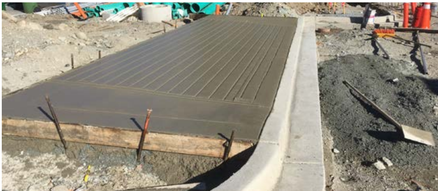
New curb and driveway ramp on the north side of Lougheed Highway, west of 225th Street.
