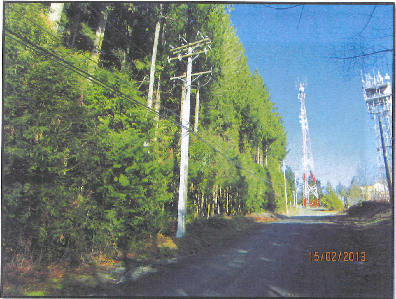
Figure 5 Example of a vulnerable wood pole power supply to critical infrastructure communication towers located on Thornhill, narrow road access and lack of water supply increase infrastructure vulnerability. Vegetation management and replacement with concrete poles could significantly improve the wildfire risk profile.
