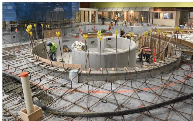
In 2019 the upgrade of the City's Leisure Centre neared completion. This facility originally opened in 1981 and these upgrades will deliver more efficient mechanical systems, modern accessibility features and improved amenities for the next generation of guests.
