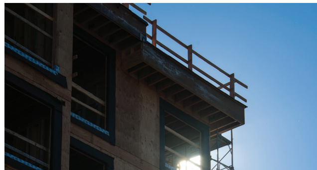
The Building Department helps ensure that construction in the City of Maple Ridge meets or exceeds all building codes. This helps protect the investment that our citizens make in their homes and businesses.
