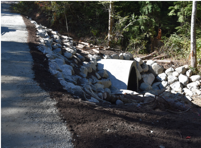
The 'Atmospheric River' in November of 2021 resulted in extensive damage to some infrastructure. This culvert located in east Maple Ridge had to be completely replaced due to the high streamflows.
