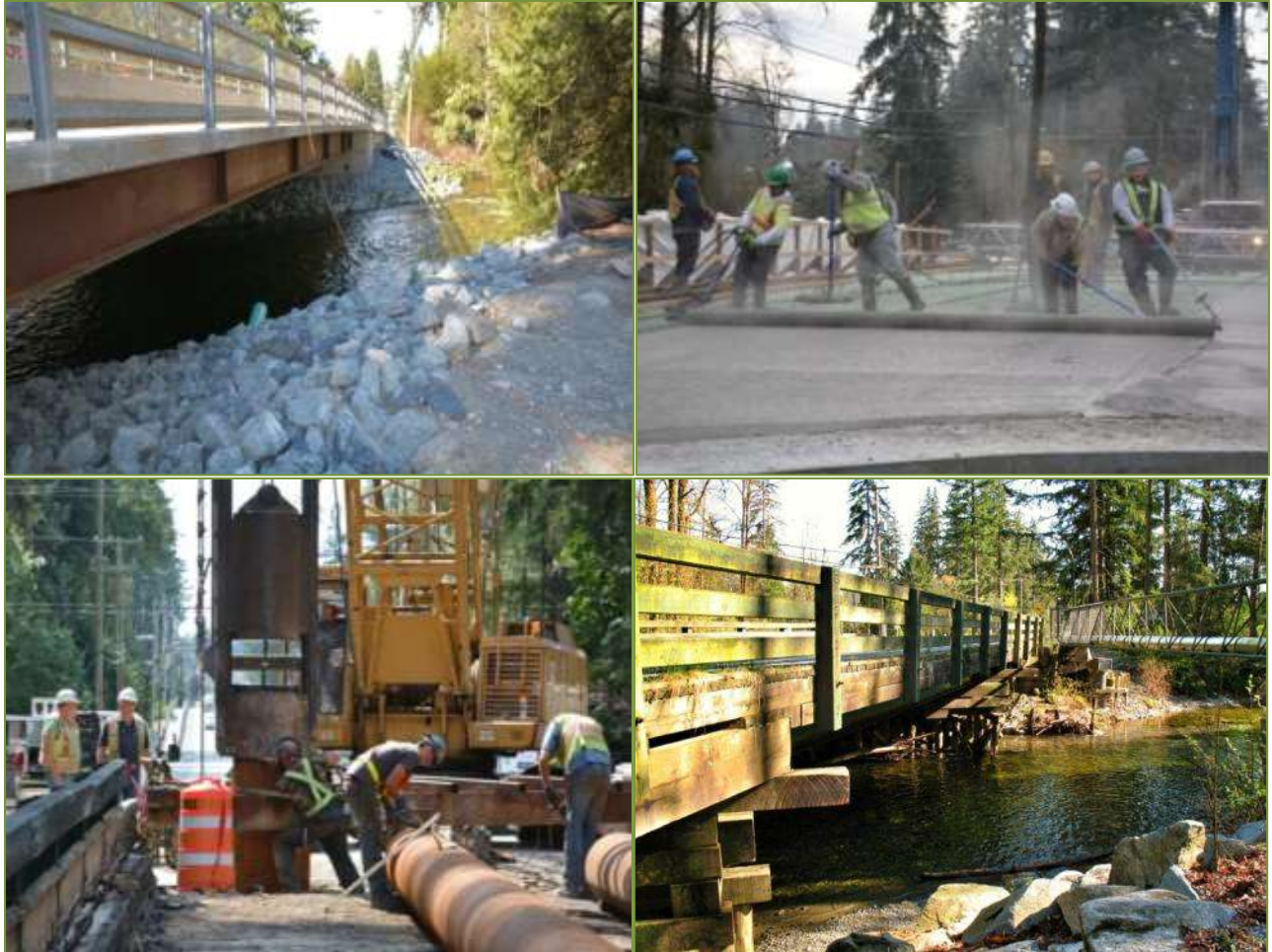
Replacement of bridge on 232 Street over the North Alouette River in the vicinity of 132 Avenue
