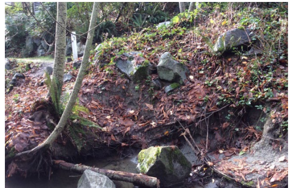
Photo 5-2: Bank Erosion @ River Rd. near River Bend Facing Southwest
