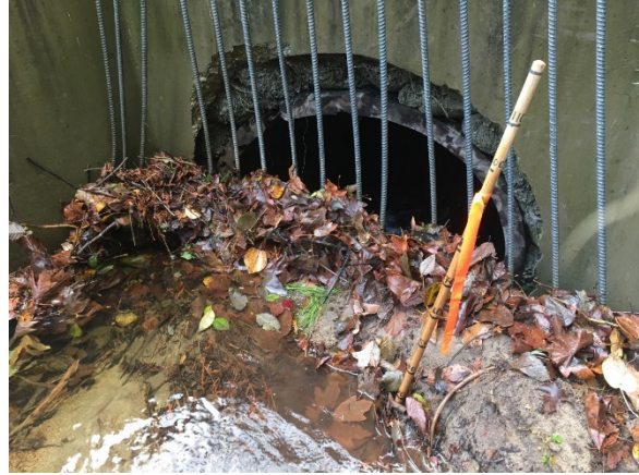
Photo C-4: Anderson Creek culvert at 232 St is an old wood stave culvert and is clogged by sediment and debris, creating a fish barrier
