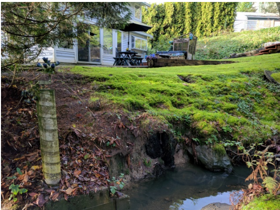
Photo A-1: Bank Erosion near Brickwood Close Facing North West
