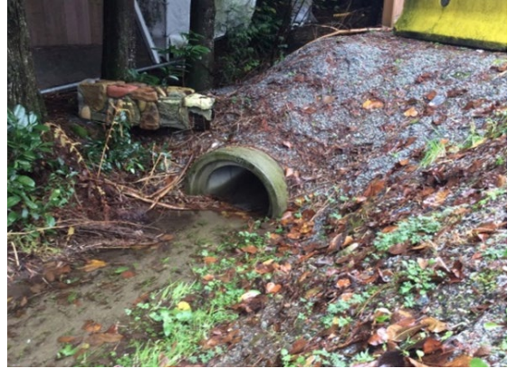
Photo 4-1: Possible Undersized Ditch Along 232 Street near North Alouette River 6
