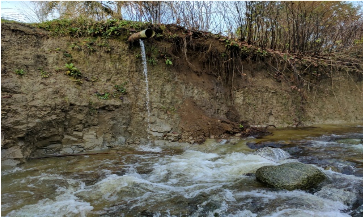
Photo A-3: Bank Erosion @ 144 Ave on Blaney Creek
