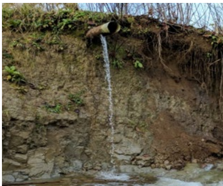
Photo 5-3: Bank Erosion on Blaney Creek near 144 Ave.
