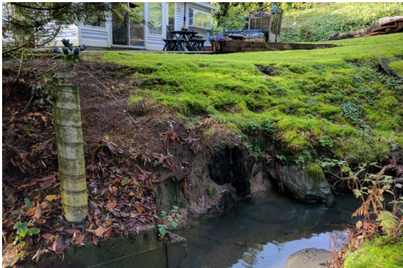
Photo 5-1: Bank Erosion near Brickwood Close Facing North West
